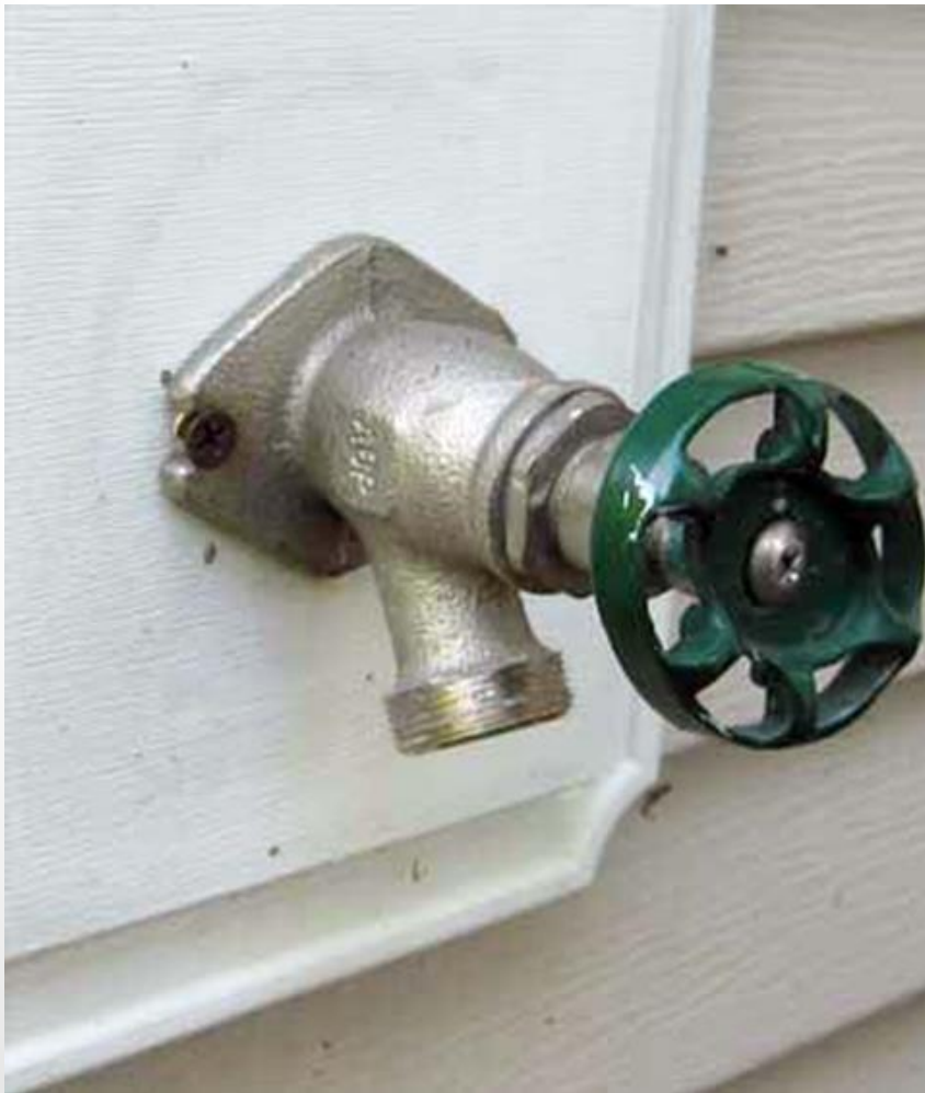
No vacuum breaker
