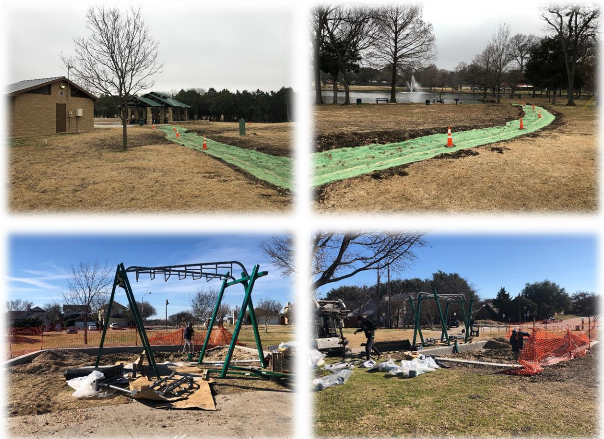
Top Row: Drainage at Lakeside Park; Bottom Row: Installation of fitness equipment at Pyburn Park
