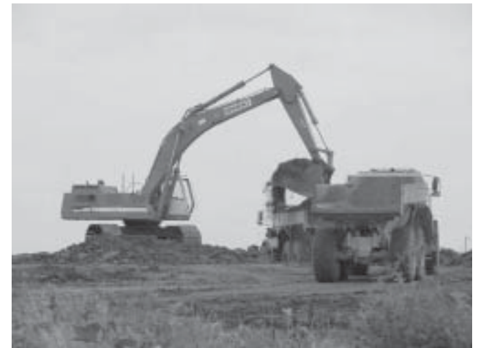
Construction has begun on the projects approved in the October 2001 bond election. Pictured is the initial site work for one of two new elementary schools. This is the site for the C.J. and Anne Hyman Elementary located in the Mt. Creek area of the district ( west section of the district boundaries ).
